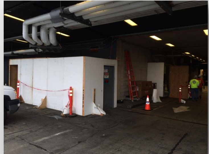
NSAT regulated materials enclosure
