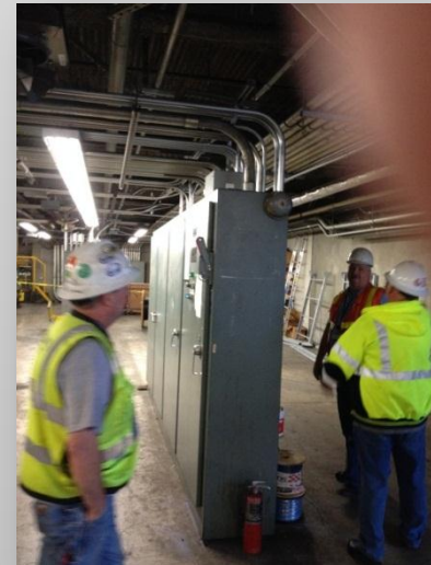
Concourse D Conveyor Motor Control Panel
