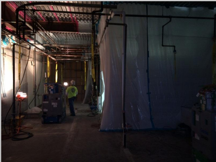
NSAT motor control panel room regulated materials enclosure
